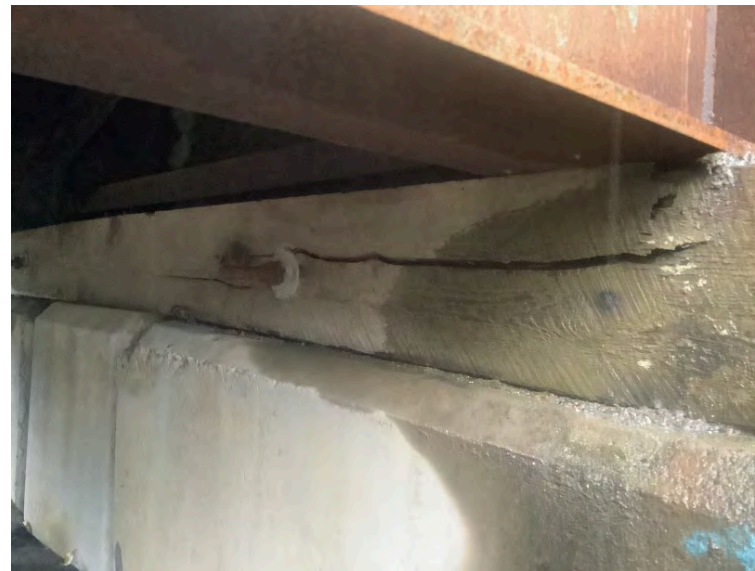
Left downstream, bearing timber crack
