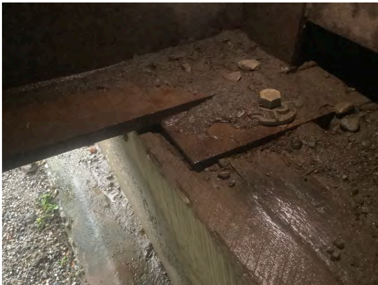
Slight crushing of bearing timber
